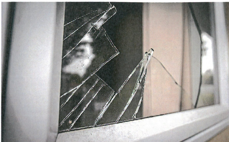
Damage by tenants is a thorny issue.
